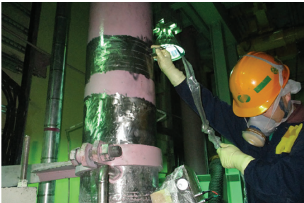
ISI services for pipes, components, and structures
