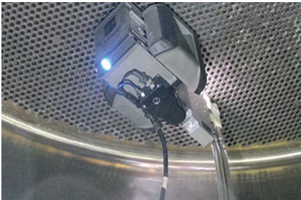
ISI services for heat exchanger tubes of a steam generator
