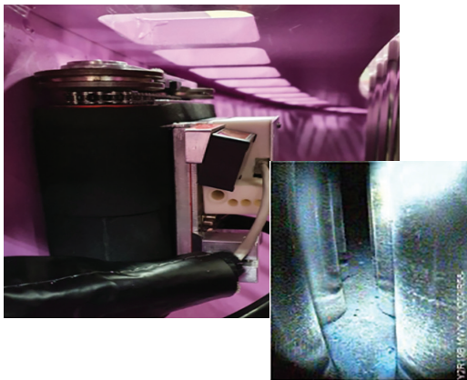
Secondary side of a steam generator In-Bundle FOSAR
