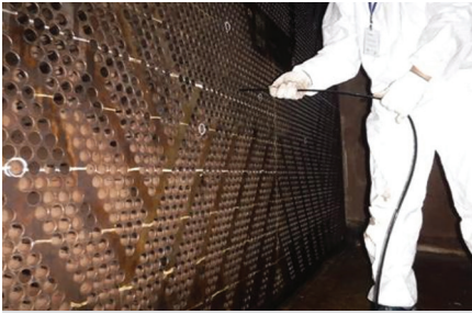
Eddy current testing services for main condenser tubes
