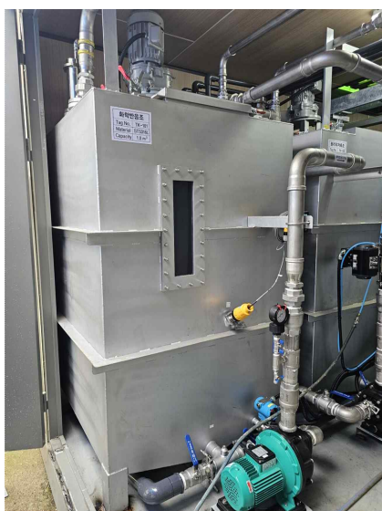
(c) Chemical reaction tank
